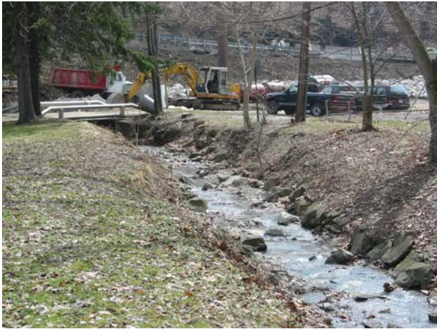
Sugar Camp Park – unnamed tributary of Dirty Camp Run Looking downstream at mild erosion problems. (Allegheny County project on Pitcairn Road underway in the background.)
