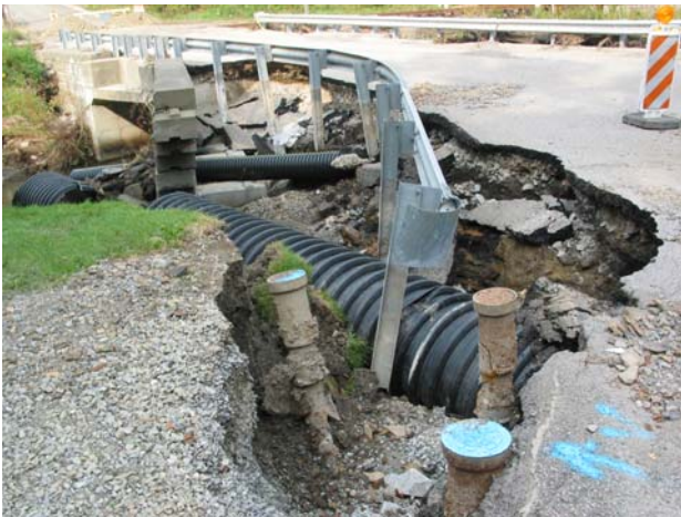
Hurricane Ivan flood damage TCWA
